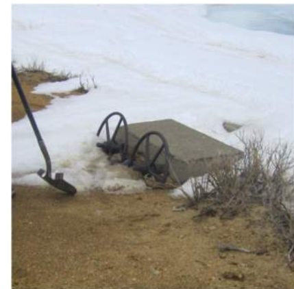
Outlet manually controlled by equipment that freezes
